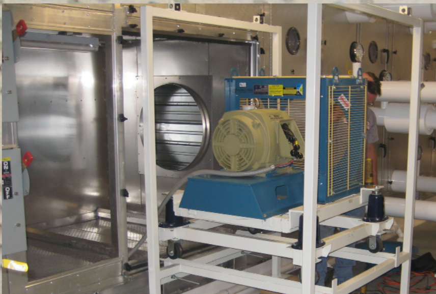
Access Panel Removed And Fan Rolled Onto Rack
