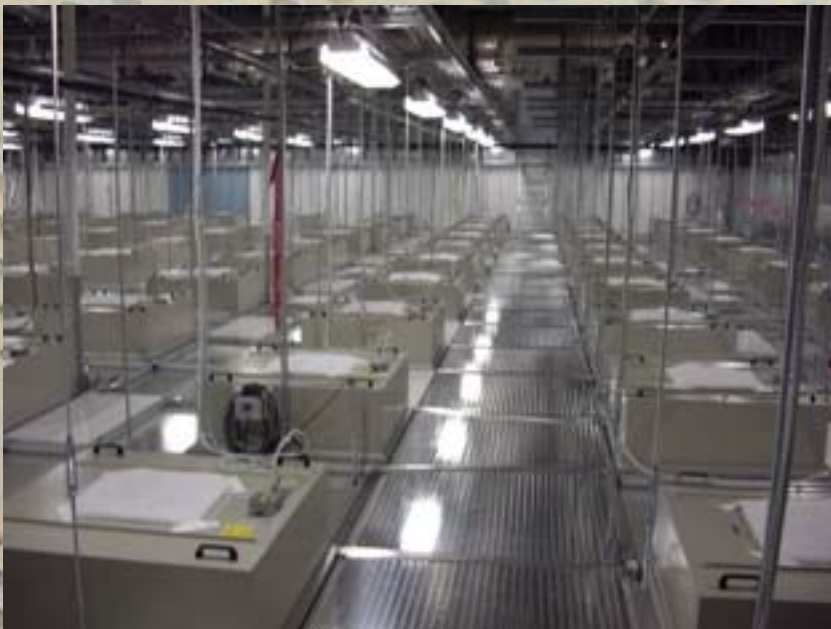
Photo of 2000 4 x 4 Fan Filter Units Installed At A Leading Microelectronic Facility
