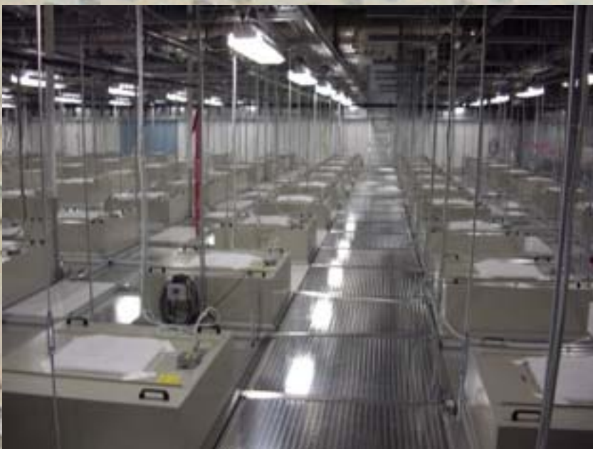
Photo of 2000 4 x 4 Fan Filter Units Installed At A Leading Microelectronic Facility
