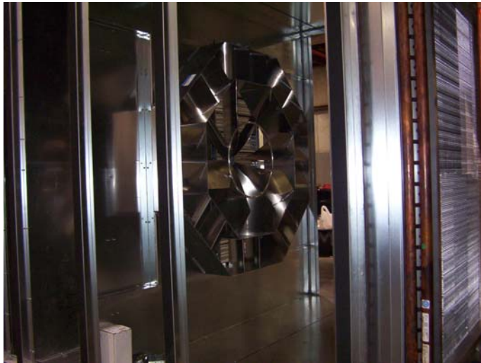
Air blender and air flow monitoring station.
